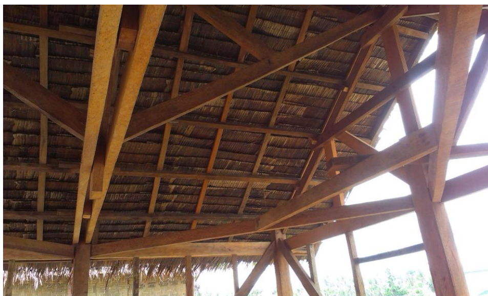
Figure 4: Roof structure (coco lumber) and nipa roofing. The nipa shingles are overlapped by 3". Project: Temporary shelters by IOM, All Hands Volunteers & Operation Blessing, Tagpuro, Leyte, Philippines. (Photo R. Dodds, Humanitarian Shelter Working Group)
