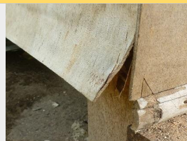
Figure 2: warping of untreated plywood, Bantayan Island, Philippines. (Photo: R. Dodds, Humanitarian Shelter Working Group Philippines 2014)
