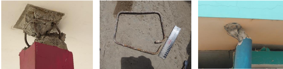
Figure 15 – Inadequate design and detailing for shear
