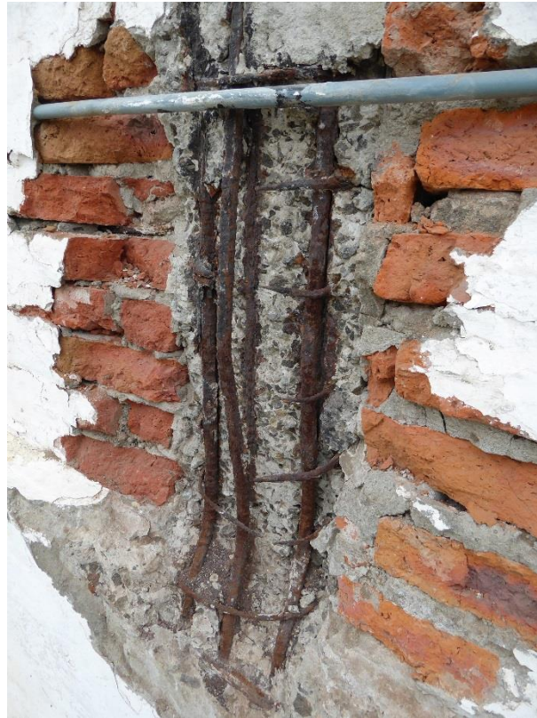
Figure 16 – Insufficient cover to rebar
