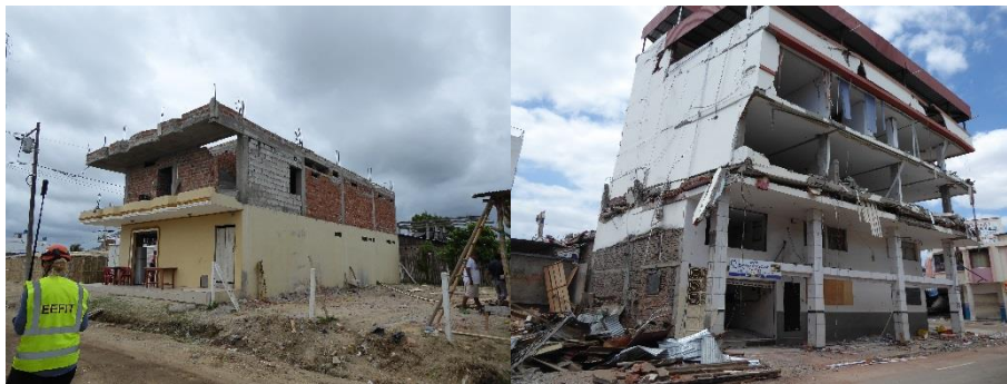
Figure 17 – Exposed reinforcement with possible inadequate lap lengths for future construction, and an upper storey soft storey failure
