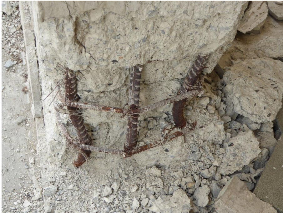
Figure 18 – Poor quality concrete
