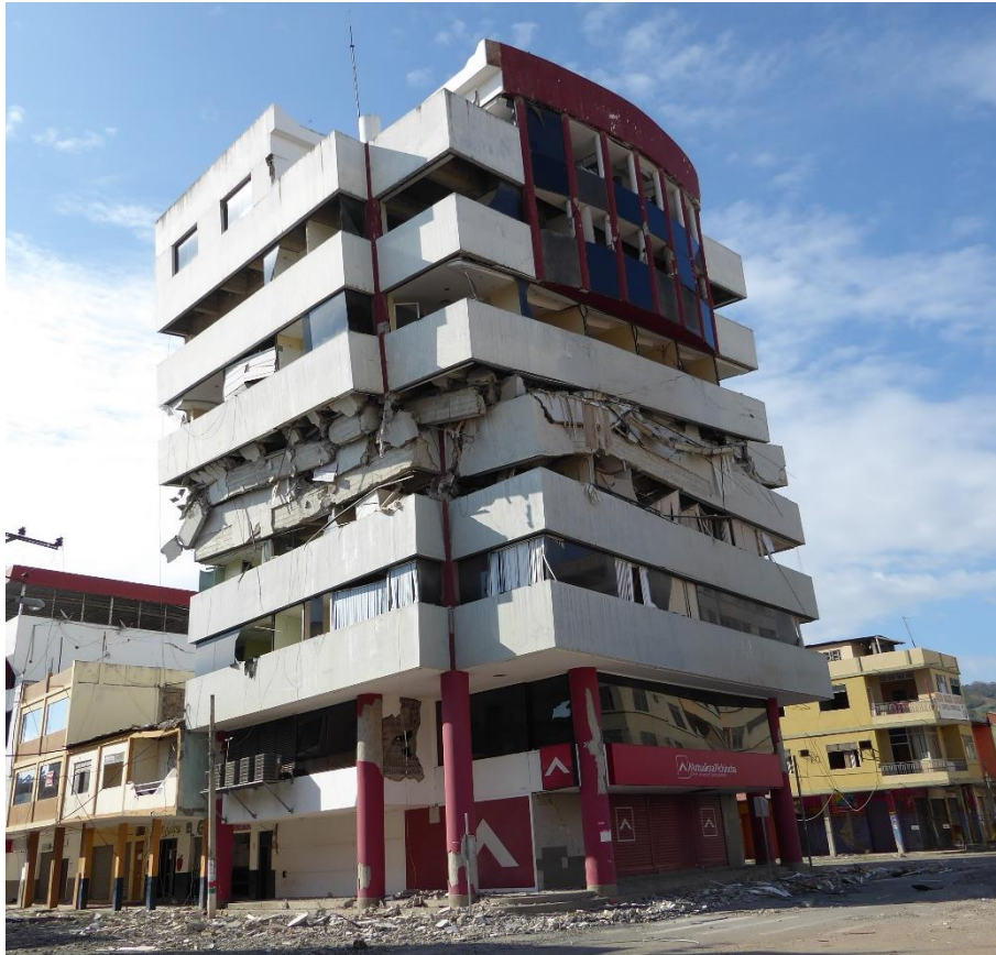
Figure 6 – Upper floor soft storey collapse on two floors in Portoviejo
