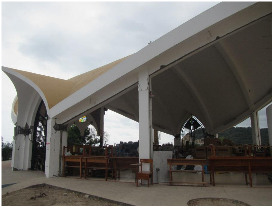
Figure 9 – Structural damage of Church in Canoa.
