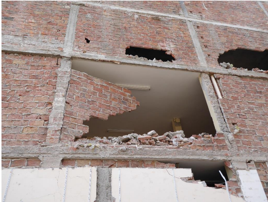
Figure 13 – Inadequate masonry infill wall design and construction
