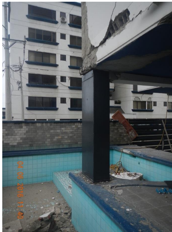
Figure 8 – Steel casing installed around ground floor columns just days before the 16 April 2016 earthquake
