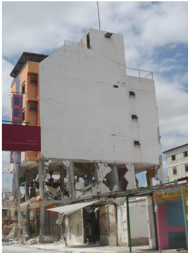
Figure 5 – Structural and non-structural damage
