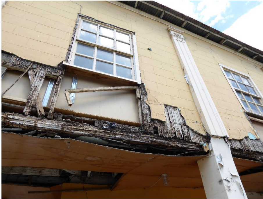
Figure 19 – Rot and damage due to insects
