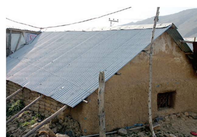
2015, T-shelter from 2008 with additional mud walling, no permanent reconstruction by this household.
